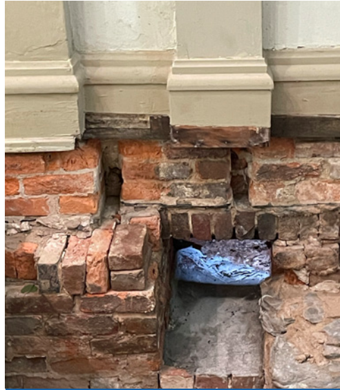
Closeup showing daylight coming through where water made its way underneath the brick and marble of St. Peter's Church beneath the statue of St. Joseph.
